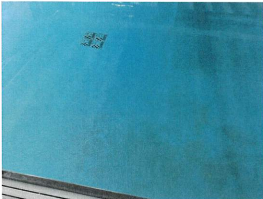
Figure 19 Program pool surface staining
