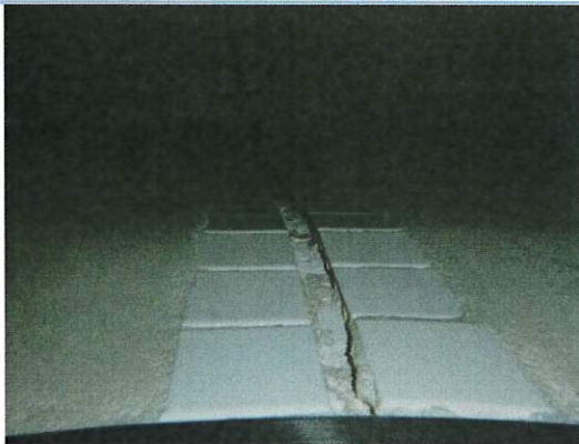
Figure 9 Cracking at pool expansion joint
