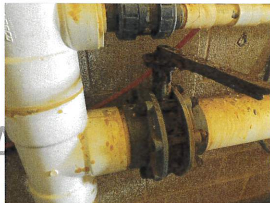
Figure 82 Lap pool piping valve corrosion
