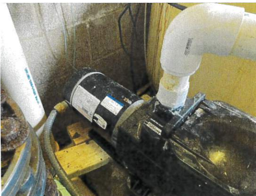
Figure 77 Program pool recirculation pump
