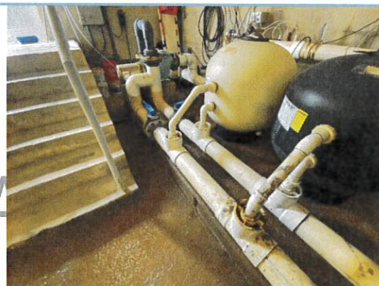
Figure 64 Outdoor pool filter piping
