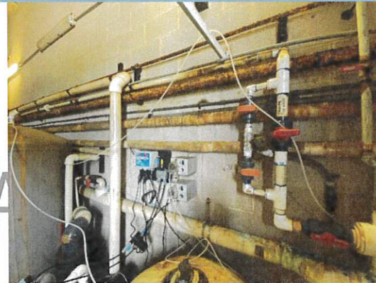
Figure 76 Program pool piping/chemical controller
