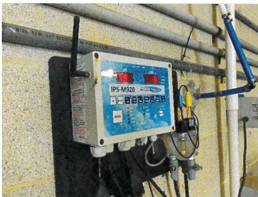
Figure 65 Outdoor pool chemical controller
