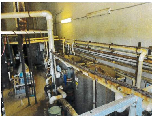
Figure 89 Lap pool recirculation piping
