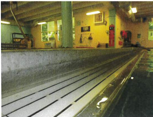
Figure 13 Lap pool perimeter overflow system
