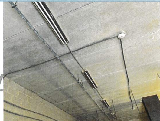
Figure 70 Mechanical room light fixture corrosion
