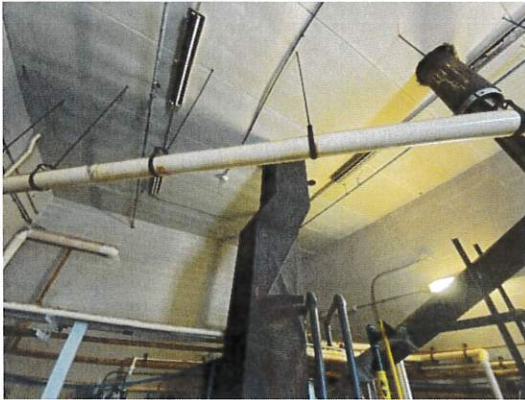
Figure 67 Pipe support corrosion
