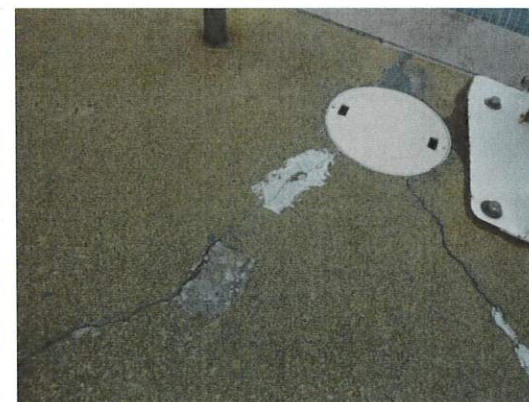
Figure 42 Pool deck repairs/cracking
