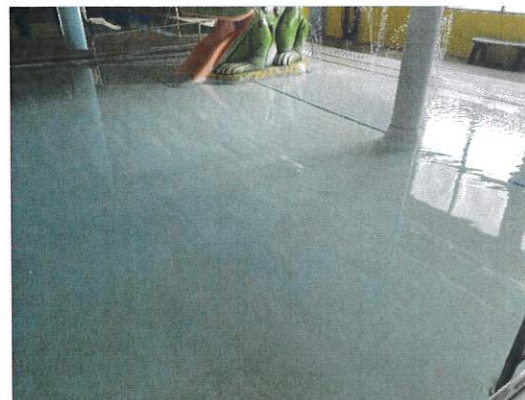
Figure 29 Program pool surface staining
