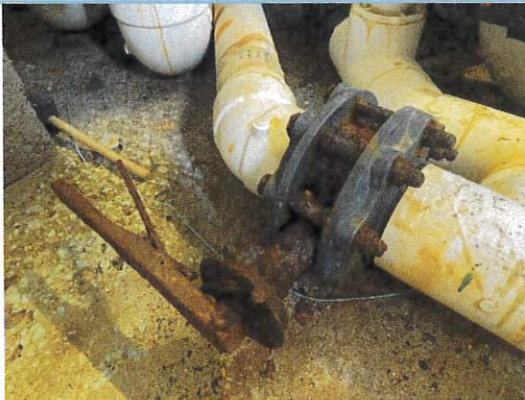
Figure 75 Program pool piping valve corrosion
