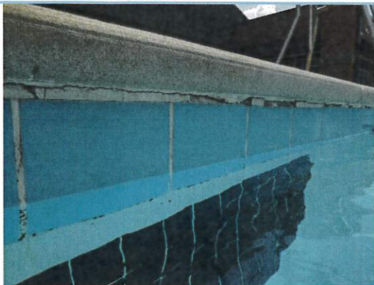
Figure 33 Mortar bed failure beneath coping stone
