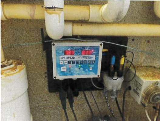
Figure 85 Lap pool chemical controller
