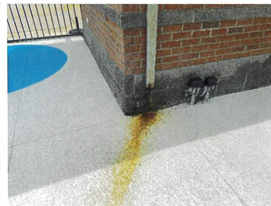
Figure 54 Deck corrosion from building water discharge
