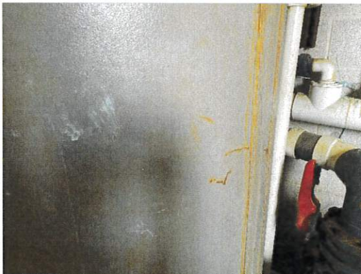
Figure 81 Lap pool filter corrosion
