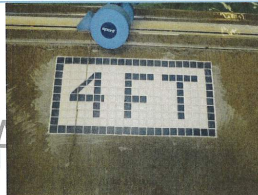
Figure 28 Program pool depth marker (cracking)
