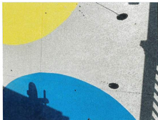
Figure 53 Cracking in spraypad surface
