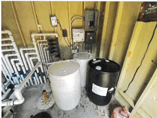
Figure 57 Spraypad chemical storage
