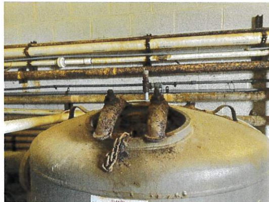
Figure 80 Lap pool filter corrosion
