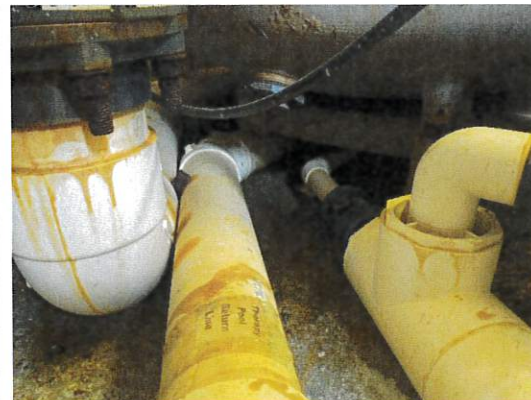
Figure 78 Program pool piping runs beneath lap pool filter
