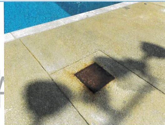
Figure 40 Diving board base corrosion
