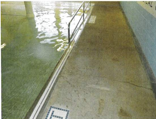
Figure 25 Program pool deck cracking
