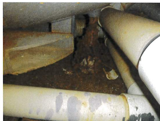
Figure 84 Lap pool filter base corrosion
