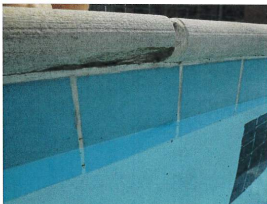
Figure 35 Gaps beneath coping stone, concrete failure
