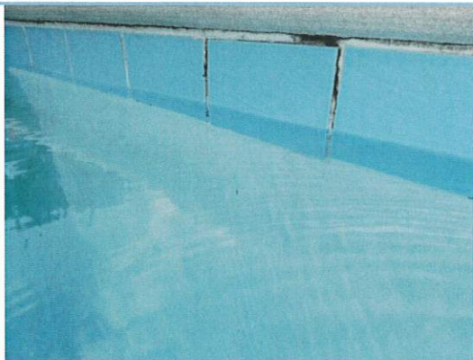
Figure 45 Missing grout in perimeter pool tile
