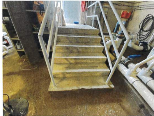
Figure 68 Mechanical room entry stairs concrete delamination
