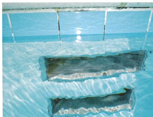
Figure 41 Missing grout in pool perimeter tile
