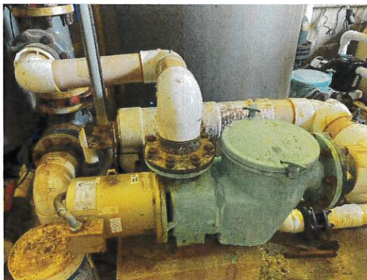
Figure 83 Lap pool recirculation pump (corrosion)
