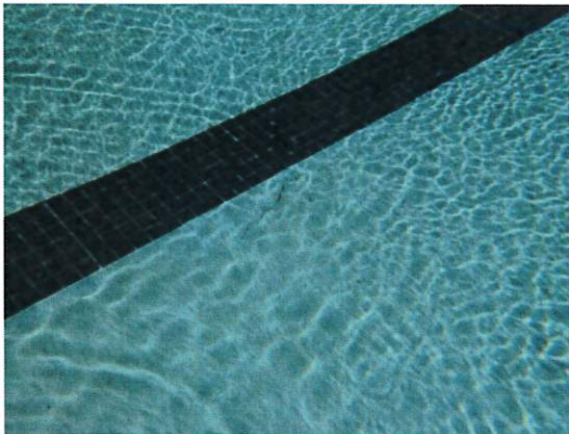
Figure 43 Pool plaster delamination
