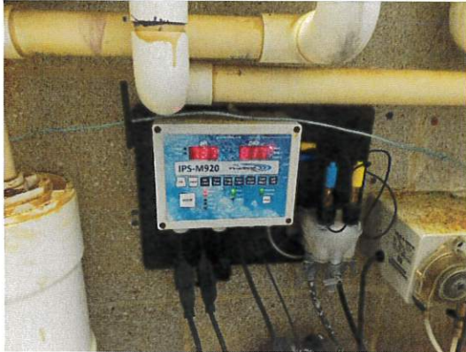
Figure 85 Lap pool chemical controller
