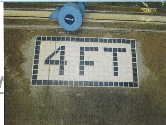
Figure 28 Program pool depth marker (cracking)
