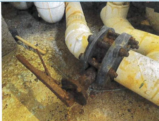
Figure 75 Program pool piping valve corrosion
