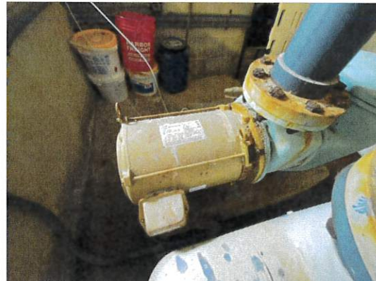
Figure 62 Outdoor pool pump/motor corrosion
