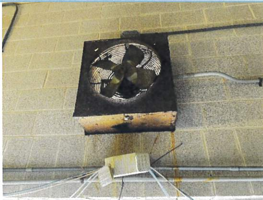
Figure 69 Mechanical room exhaust fan corrosion
