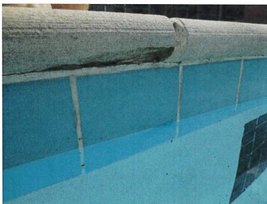
Figure 35 Gaps beneath coping stone, concrete failure
