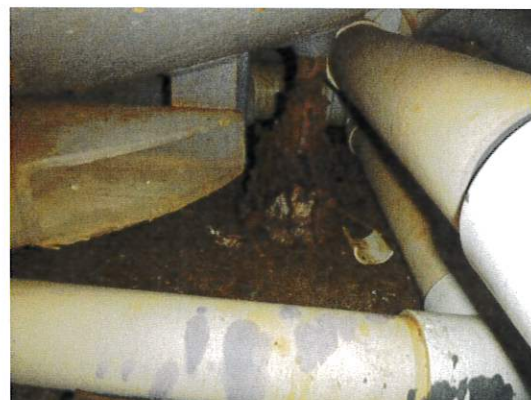
Figure 84 Lap pool filter base corrosion
