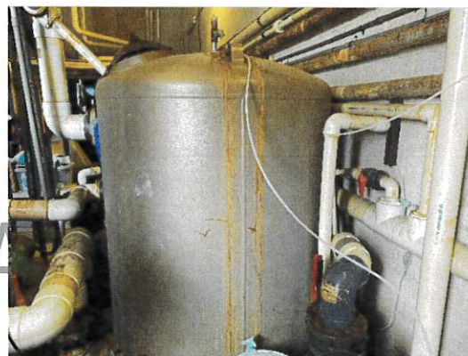
Figure 88 Lap pool chemical feed line
