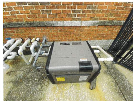
Figure 72 Indoor pool heater
