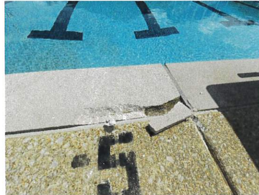
Figure 38 Broken/chipped coping stone
