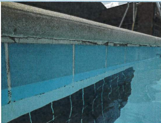
Figure 33 Mortar bed failure beneath coping stone
