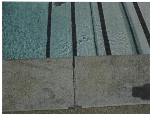
Figure 32 Coping stone missing grout/mortar
