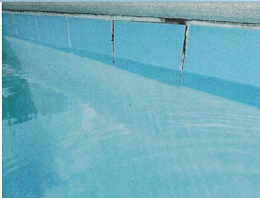
Figure 45 Missing grout in perimeter pool tile
