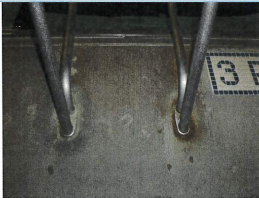
Figure 15 Lap pool ladder grab rails
