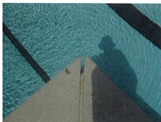
Figure 36 Coping stone missing grout/mortar
