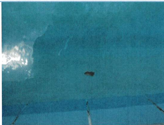
Figure 39 Hole in pool's plaster surface
