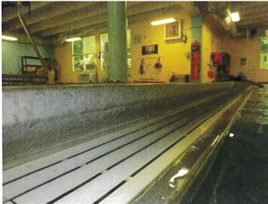
Figure 13 Lap pool perimeter overflow system
