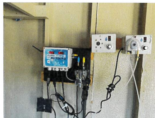
Figure 60 Spraypad chemical controller
