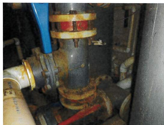
Figure 90 Lap pool piping connection corrosion
