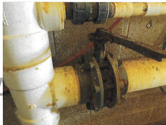
Figure 82 Lap pool piping valve corrosion
