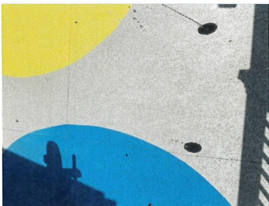
Figure 53 Cracking in spraypad surface
