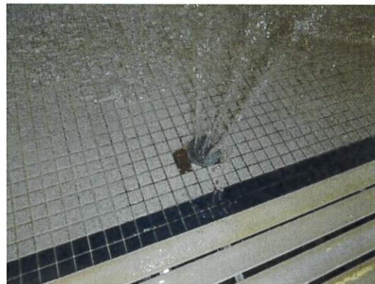
Figure 20 Program pool missing tile
