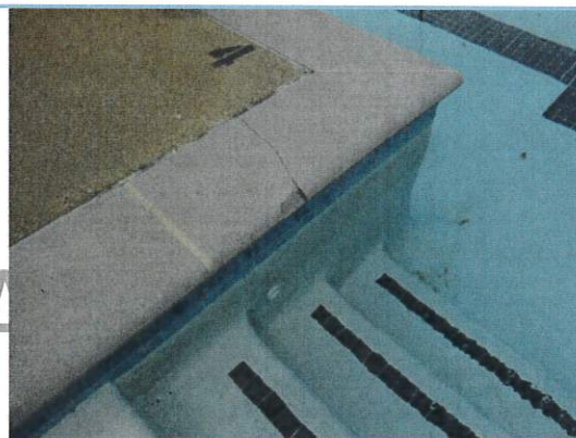
Figure 34 Chipped and cracking coping stone
