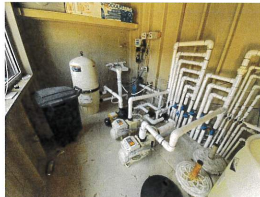
Figure 56 Spraypad recirculation system
