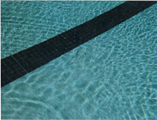
Figure 43 Pool plaster delamination
