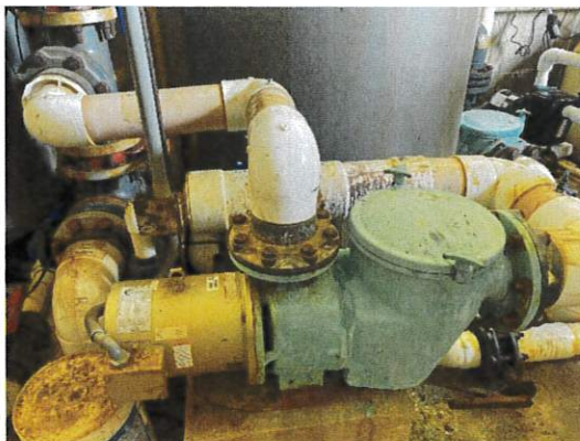
Figure 83 Lap pool recirculation pump (corrosion)
