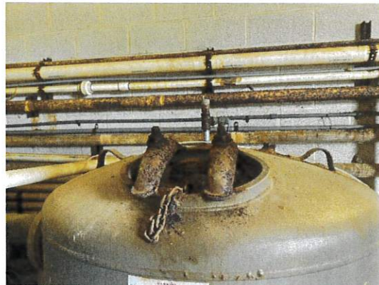
Figure 80 Lap pool filter corrosion
