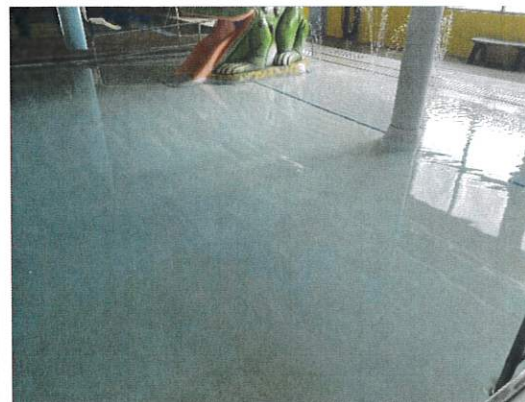
Figure 29 Program pool surface staining
