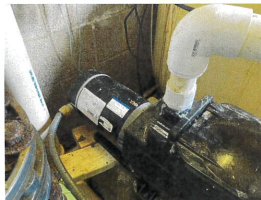
Figure 77 Program pool recirculation pump
