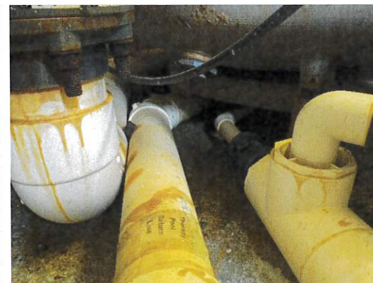
Figure 78 Program pool piping runs beneath lap pool filter
