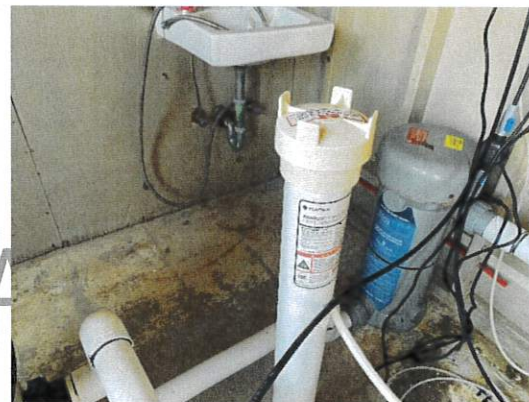
Figure 58 Spraypad chemical feeder and UV system
