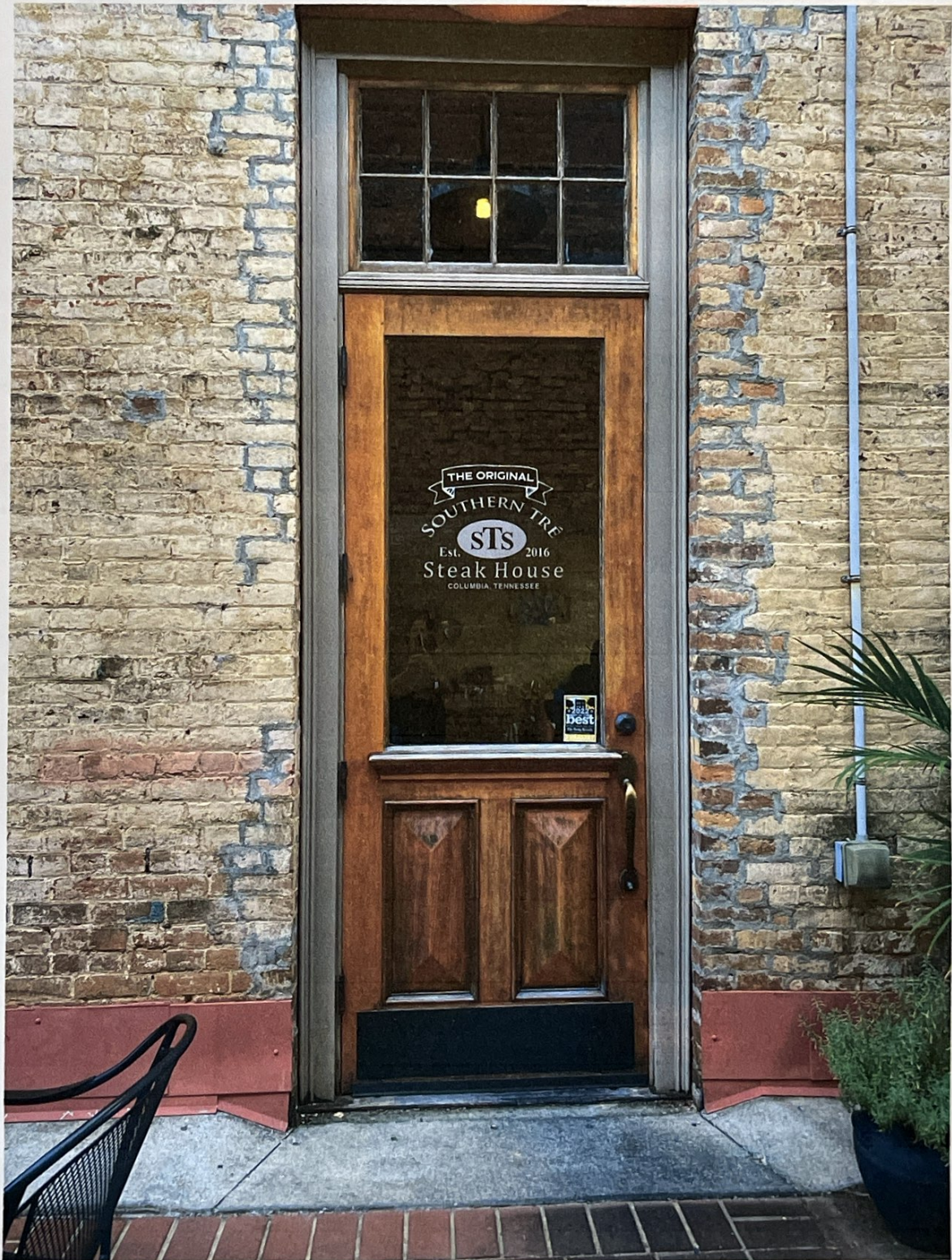
Example of proposed newly-altered door style with one-glass panel and business logo on glass.
