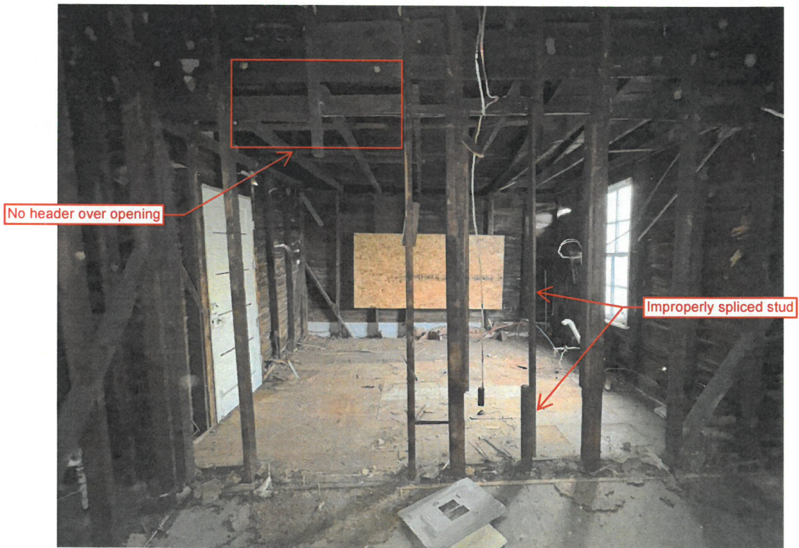
Picture 11: No Header and Improperly Spliced Studs
