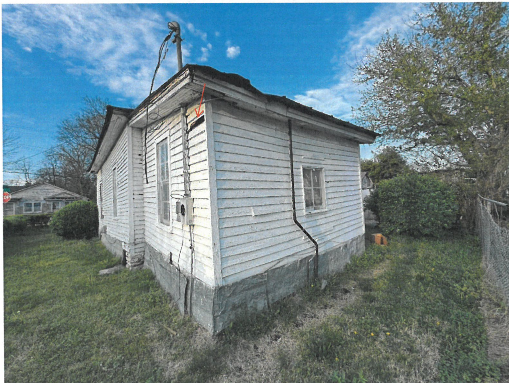
Picture 5: Deteriorated Exterior Siding/Sheathing
