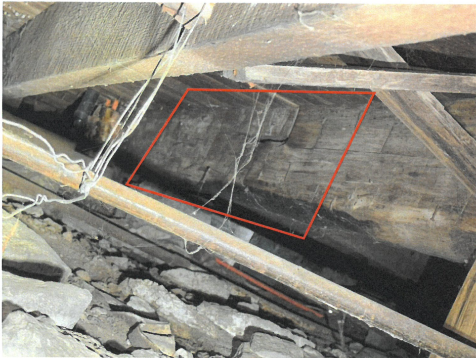
Picture 32: Splice in Main Beam Away from Support
