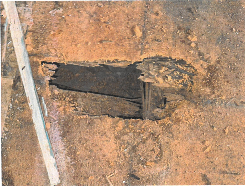
Picture 19: Deteriorated Subfloor
