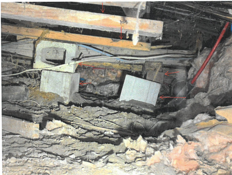
Picture 30: Haphazard Support of Floor Framing at Northeast Portion of Home
