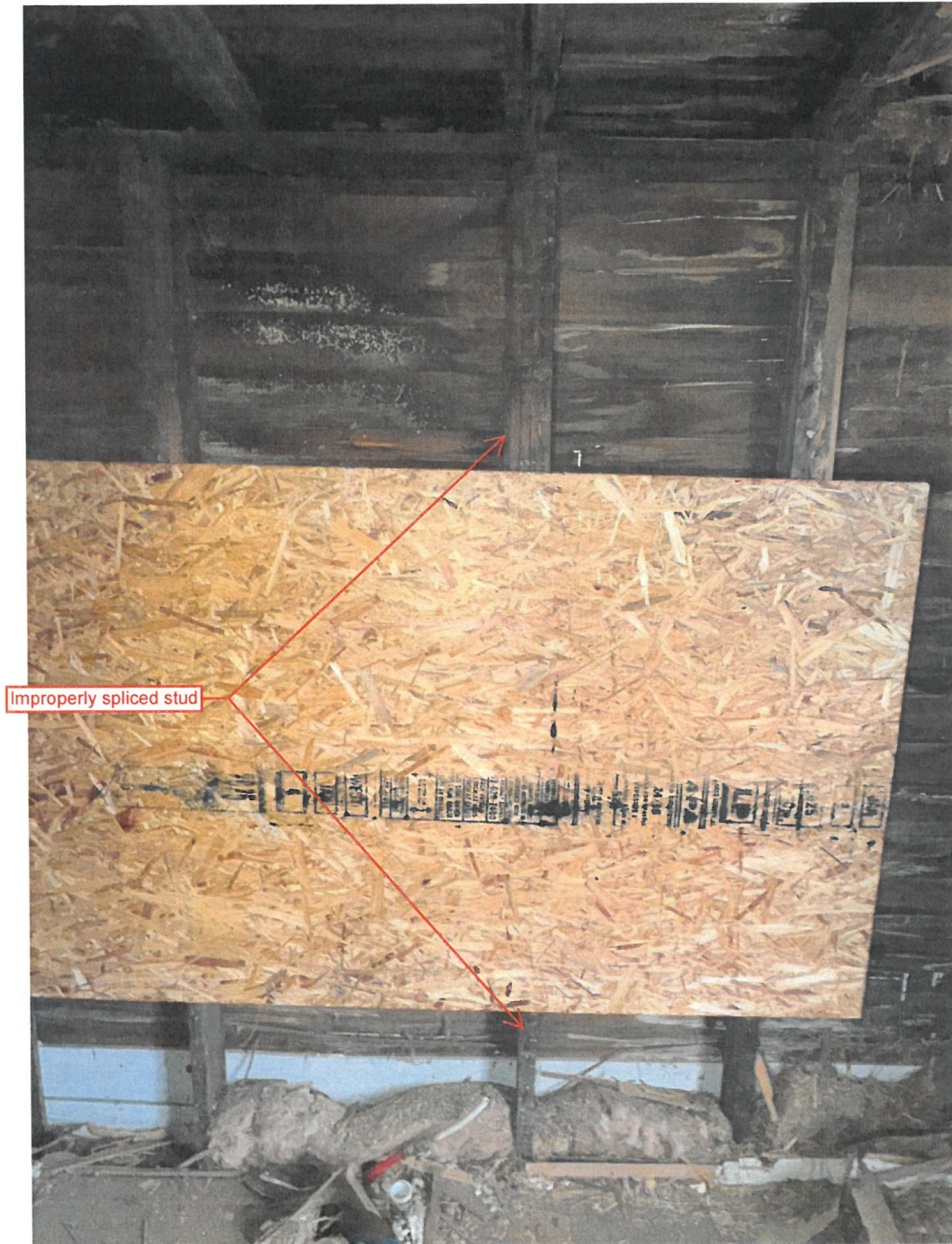
Picture 12: Improperly Spliced Studs
