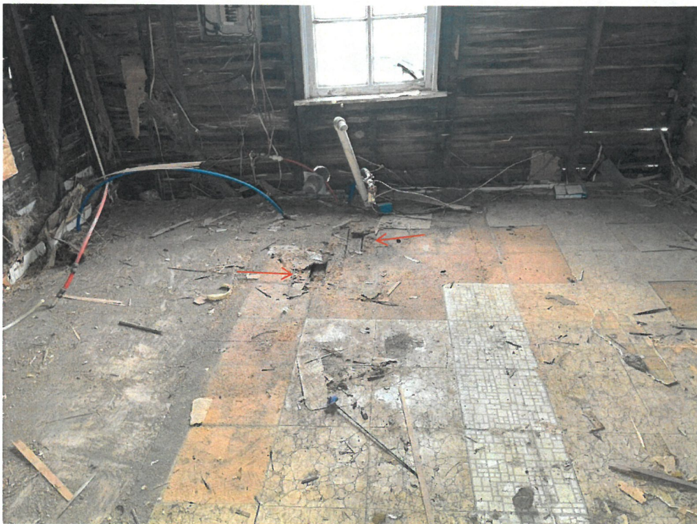
Picture 14: Deteriorated Subfloor
