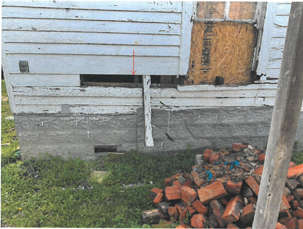
Picture 6: Deteriorated Exterior Siding/Sheathing
