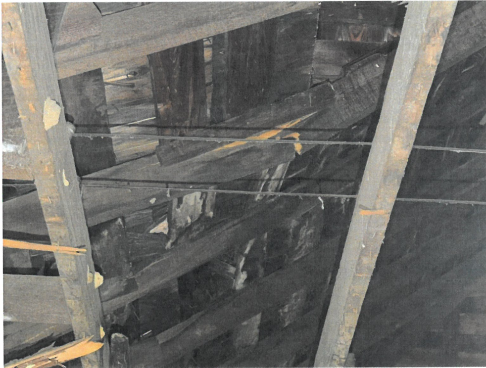
Picture 23: Fractured Rafter, Water Damaged Sheathing
