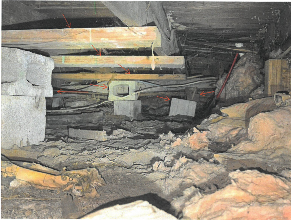
Picture 25: Haphazard Support of Floor Framing at Northeast Portion of Home
