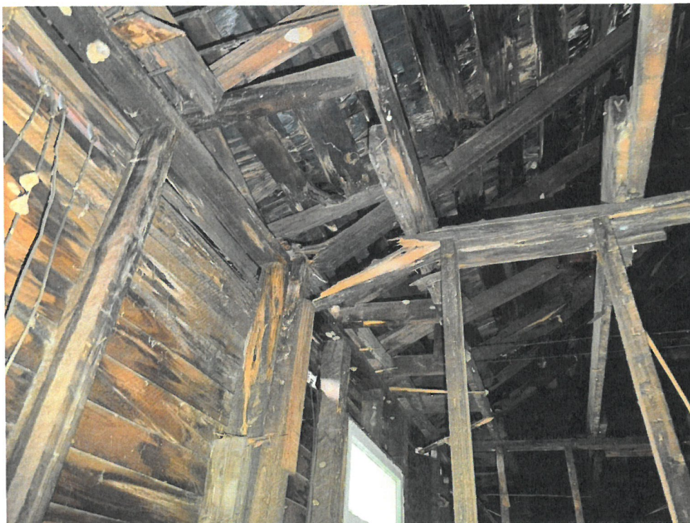
Picture 24: Fractured Framing, Water Damaged Sheathing and Lumber
