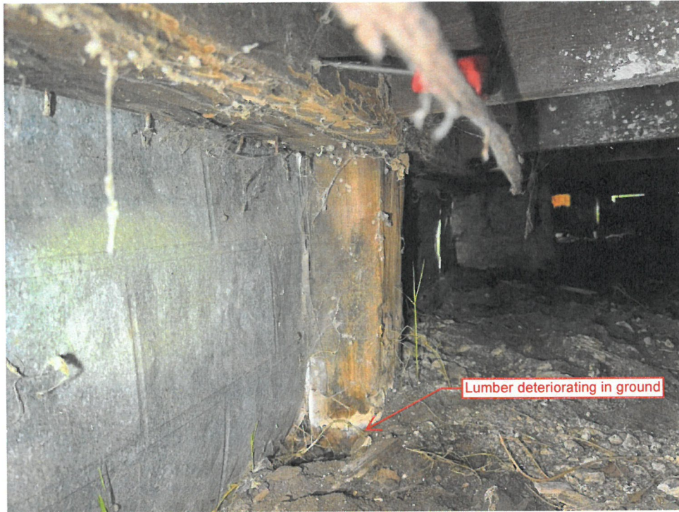
Picture 29: Post in Ground, Deterioration Evident
