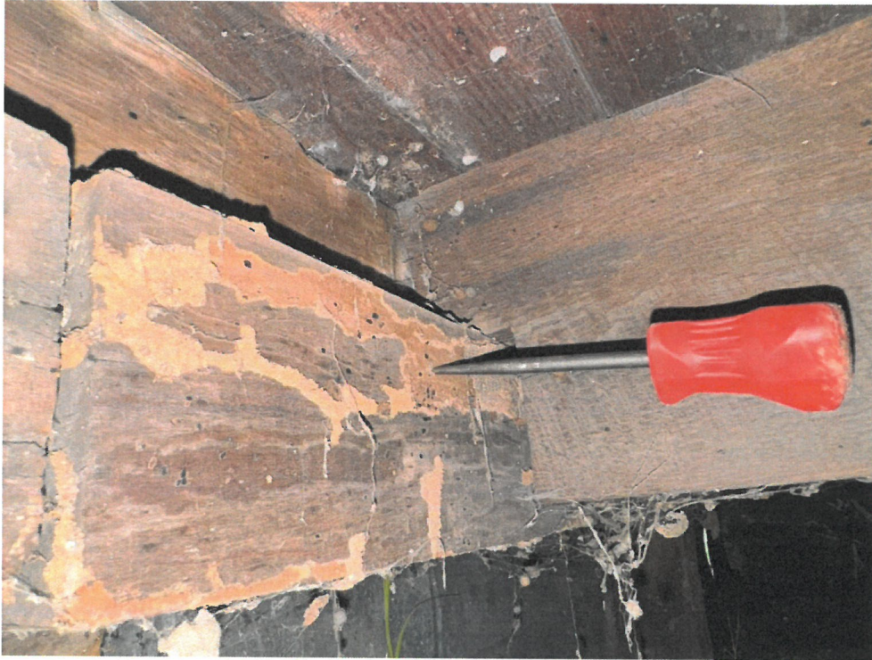
Picture 27: Excessively Notched Joists, WDI Damaged Framing
