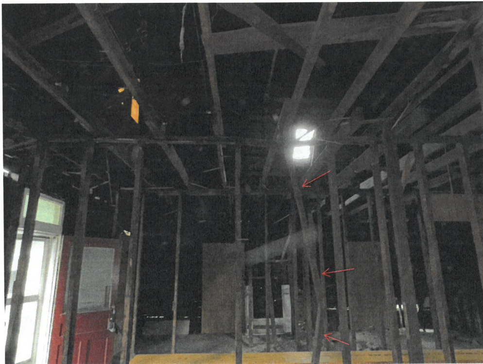
Picture 20: Failed Stud
