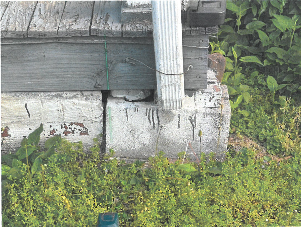
Picture 4: Settlement and Downspout Discharging at Face of Foundation
