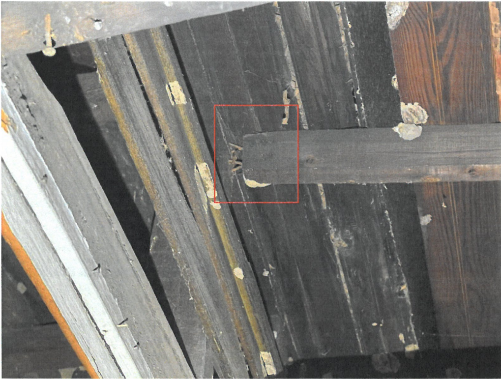
Picture 8: Poor Rafter Connectivity
