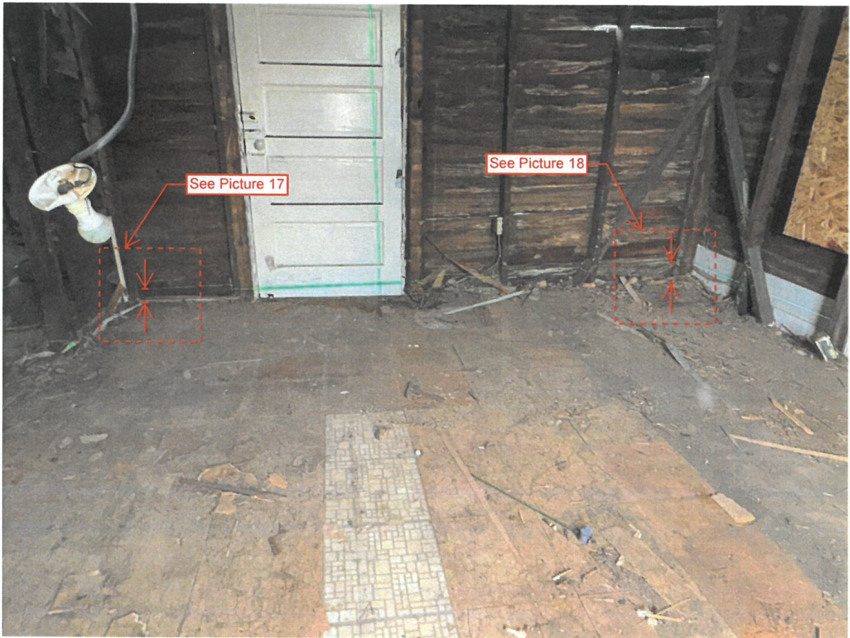
Picture 16: Sagging Floor
