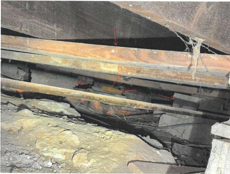
Picture 31: Haphazard Support of Floor Framing at Northeast Portion of Home
