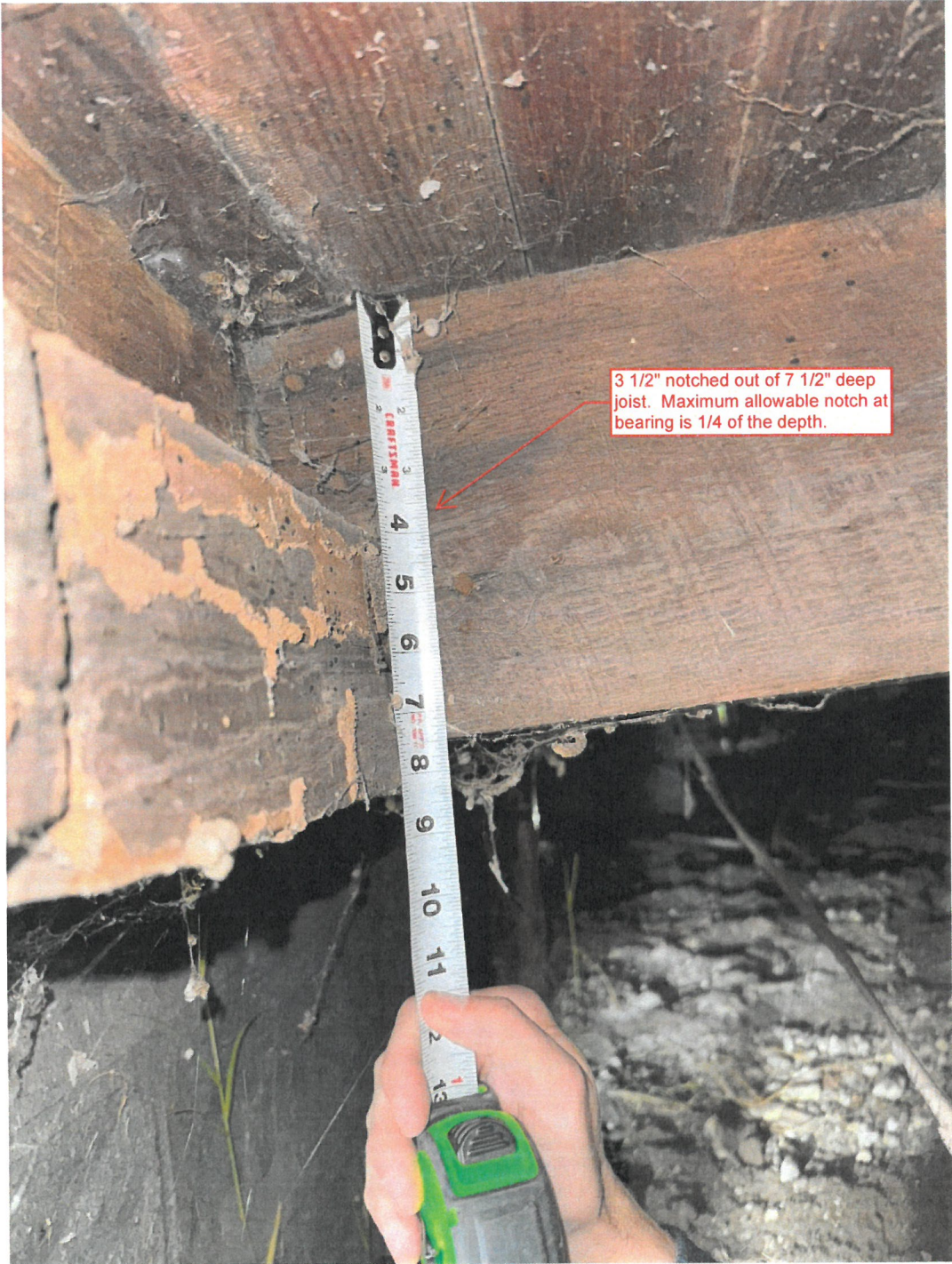
Picture 26: Excessively Notched Joists, WDI Damaged Framing
