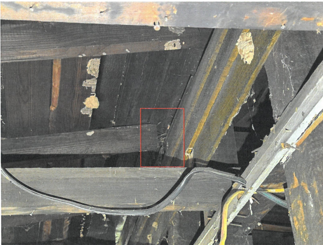
Picture 9: Poor Rafter Connectivity
