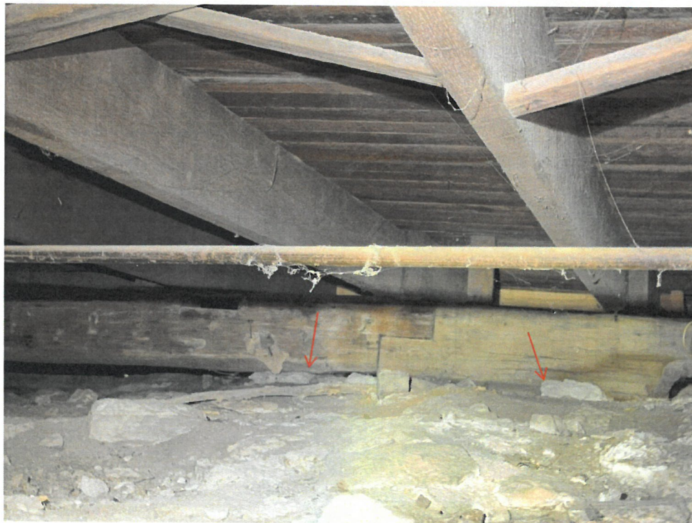
Picture 28: Main Beam Almost Touching Ground
