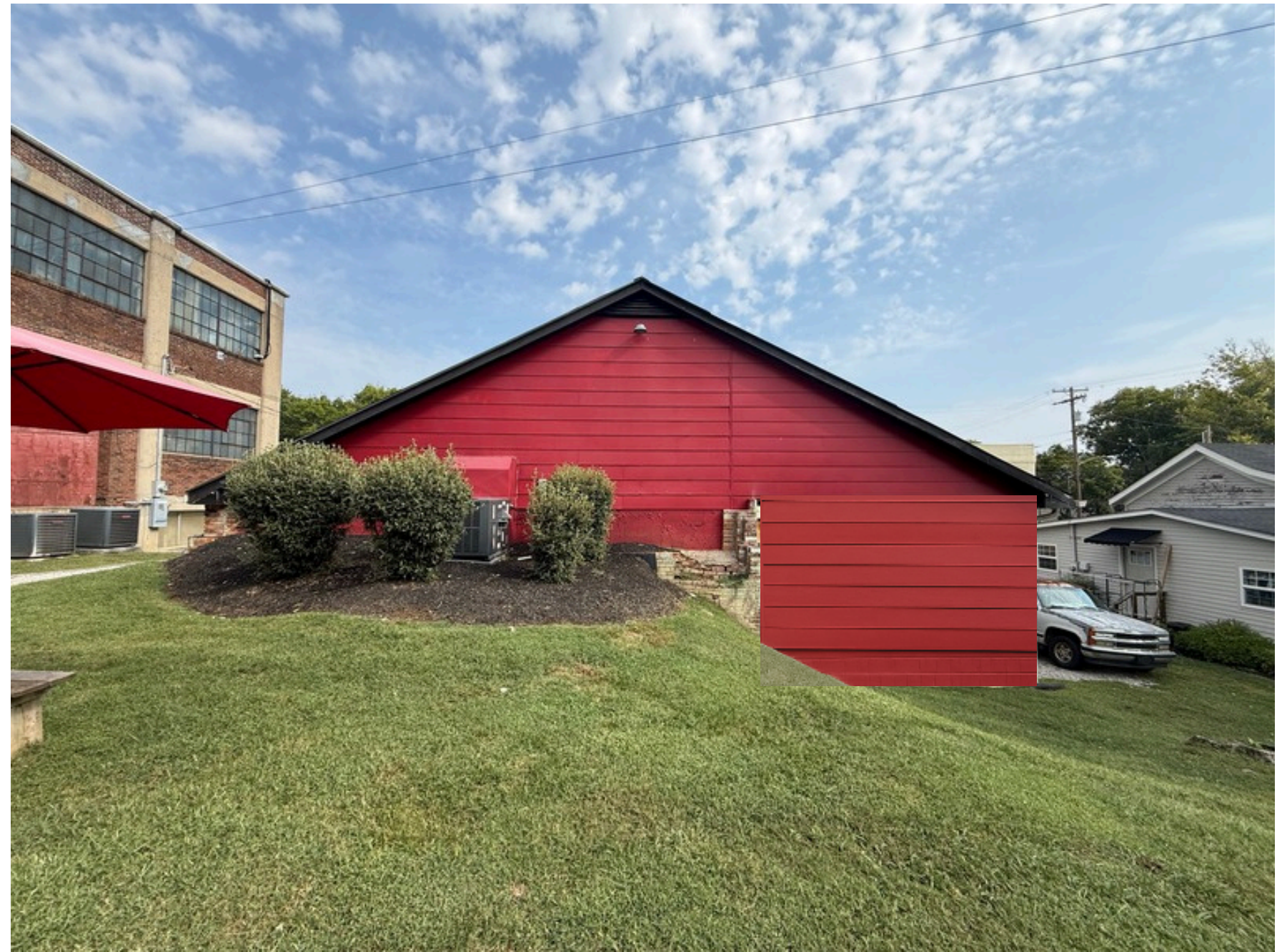
Shown with wall extended to screen boiler equipment in the back of the carport, match existing siding
