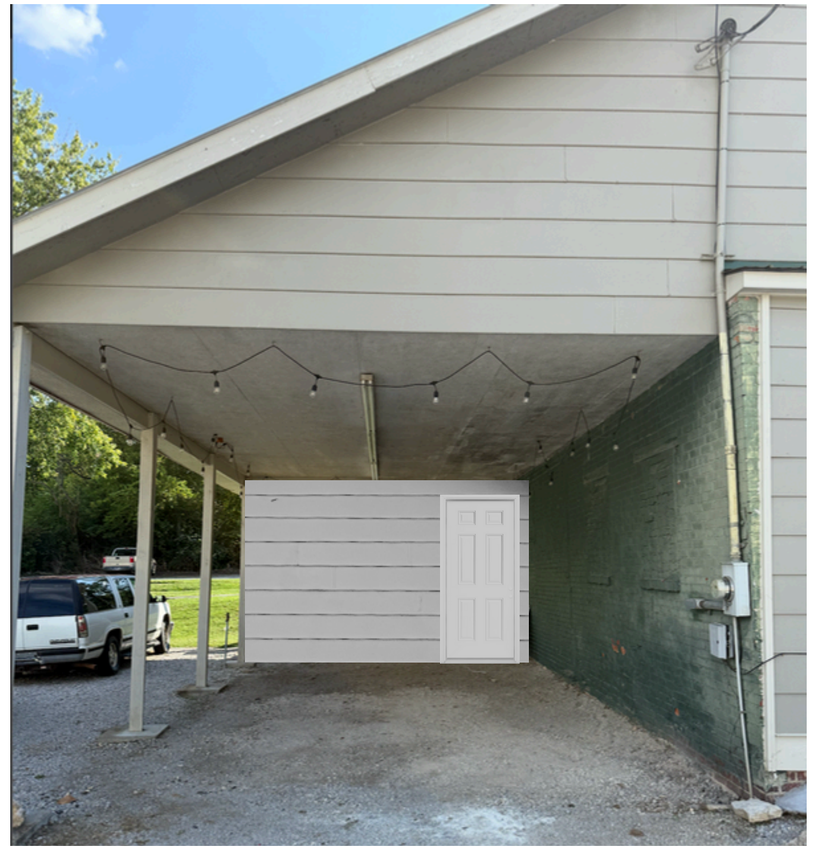
Create walls to match existing siding around the back area. This will shield the new boiler on all 3 exposed sides. There will be 2 fixed louvers on the left wall and a door on the front wall.
