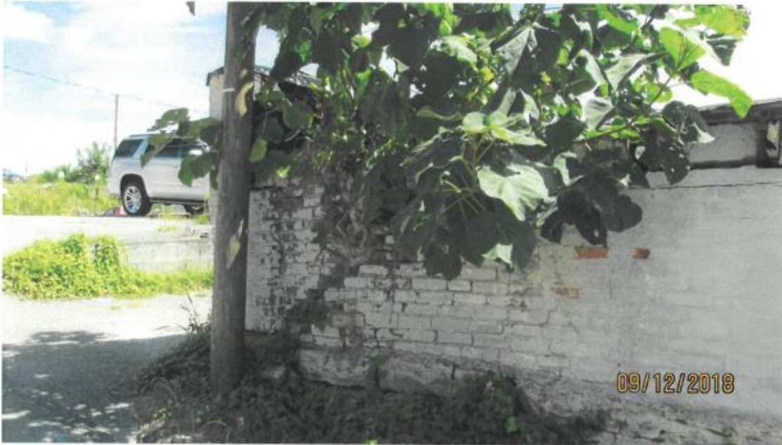
Photo #9: Damaged walls bowing out of plane
