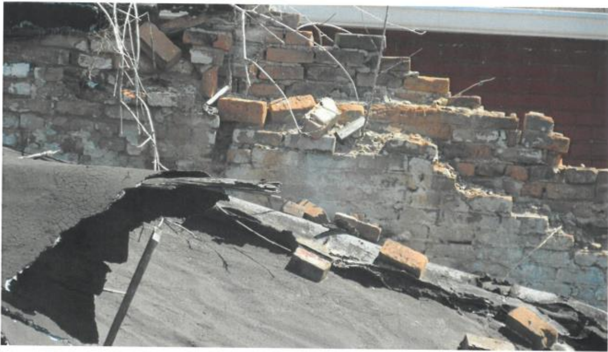
Photo #13: Collapsed roof and damaged wall
