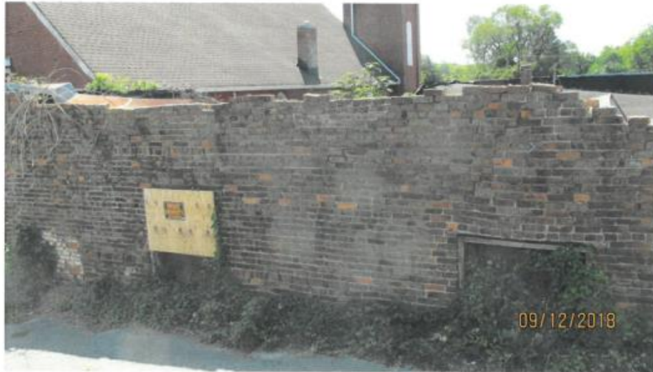
Photo #15: Severely damaged rear brick wall
