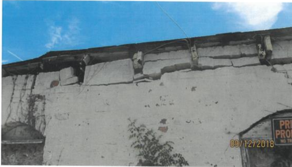
Photo #8: Damaged roof framing, brick walls, roofing.
