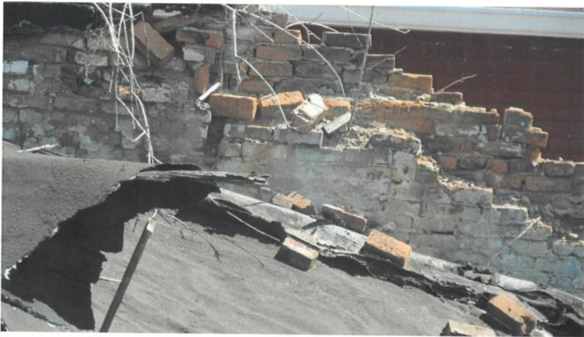
Photo #13: Collapsed roof and damaged wall
