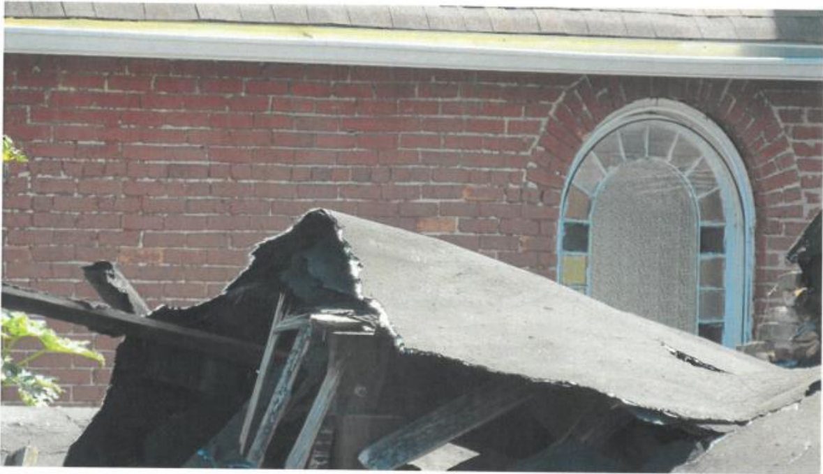
Photo #12: Collapsed roof
