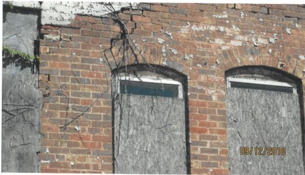
Photo #5: Cracking in front exterior wall, damaged window frames
