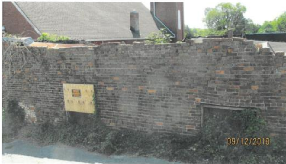
Photo #15: Severely damaged rear brick wall
