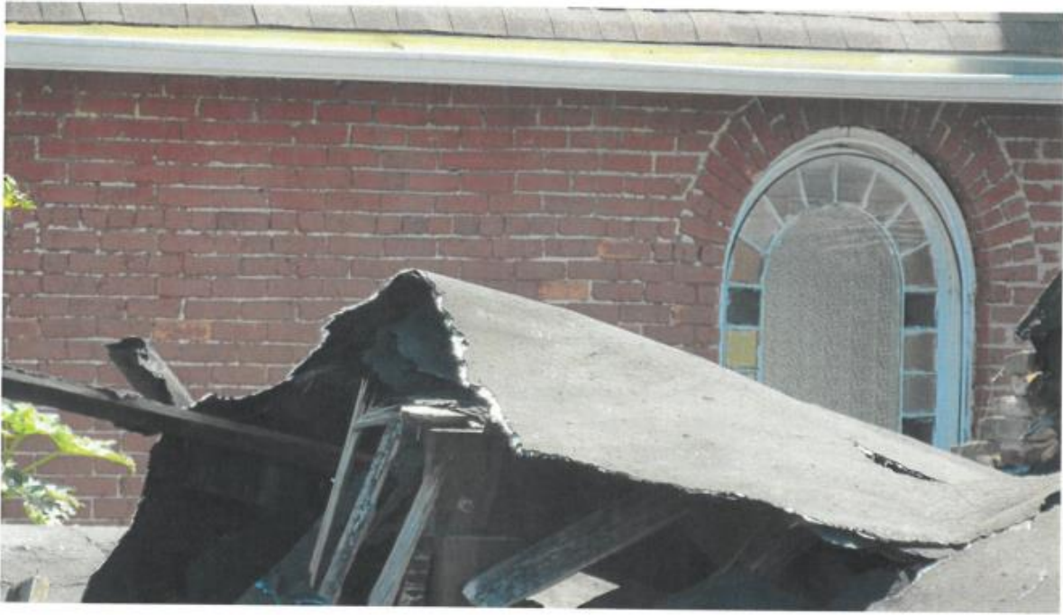
Photo #12: Collapsed roof
