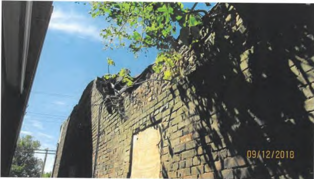
Photo #19: Damaged wall on right side
