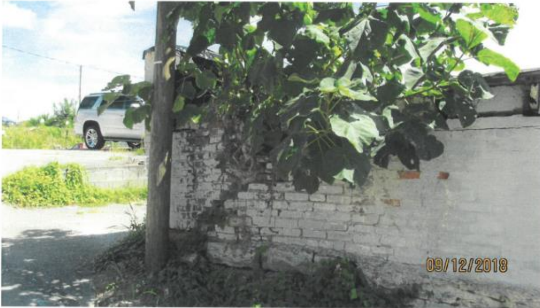
Photo #9: Damaged walls bowing out of plane
