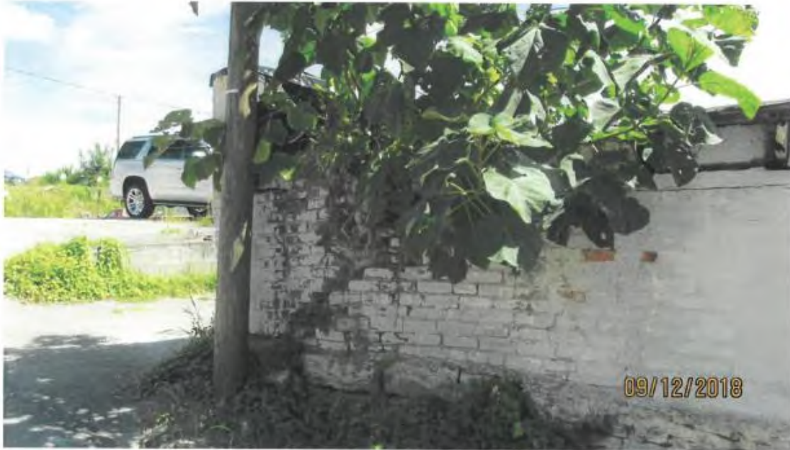
Photo #9: Damaged walls bowing out of plane
