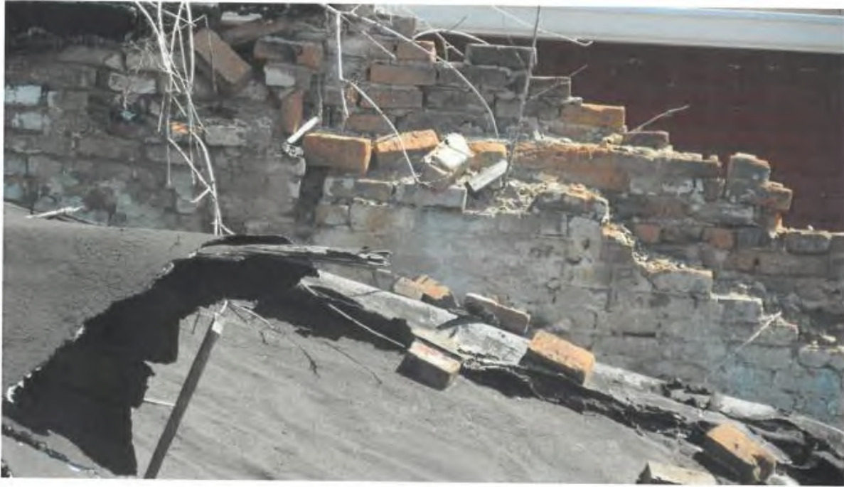
Photo #13: Collapsed roof and damaged wall
