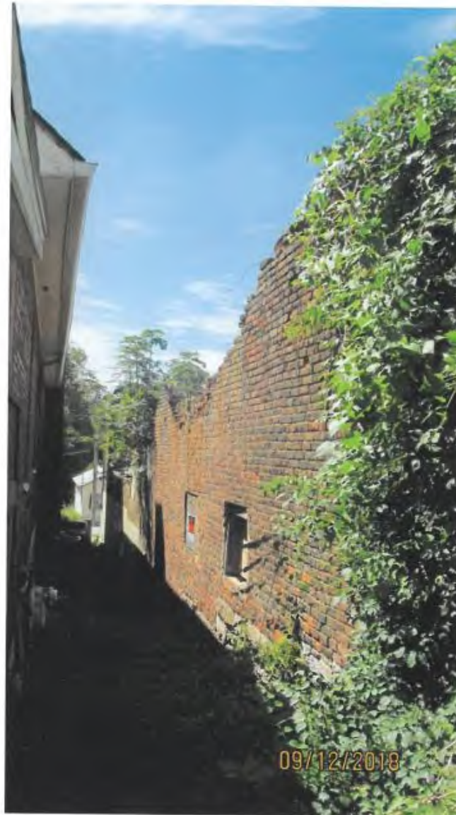
Photo #17: Damaged right side wall
