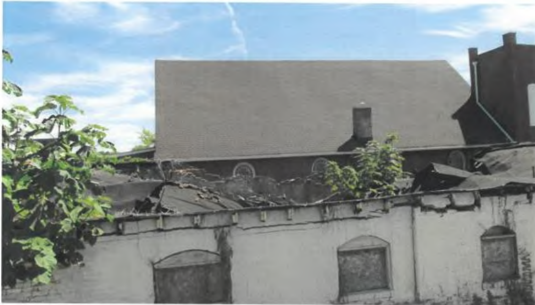
Photo #11: Collapsed roof and damage walls
