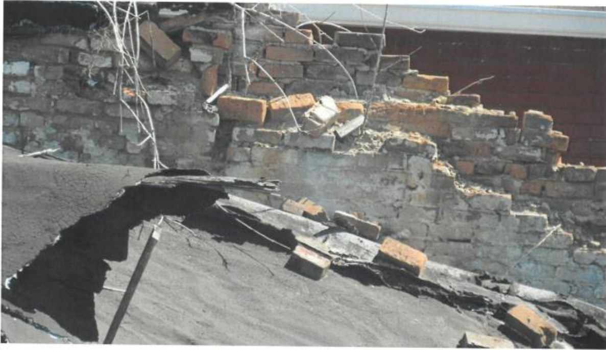
Photo #13: Collapsed roof and damaged wall
