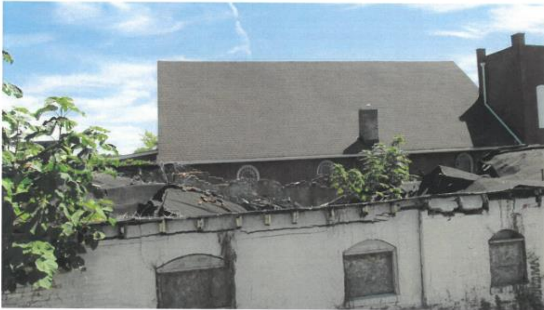
Photo #11: Collapsed roof and damage walls
