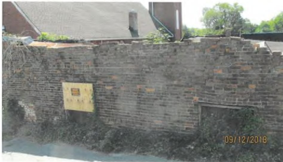
Photo #15: Severely damaged rear brick wall
