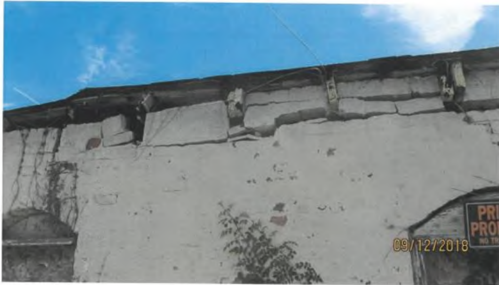
Photo #8: Damaged roof framing, brick walls, roofing.
