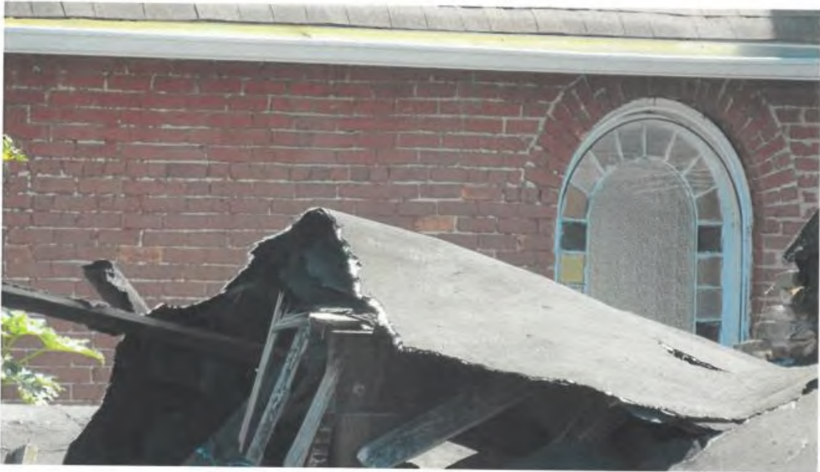
Photo #12: Collapsed roof
