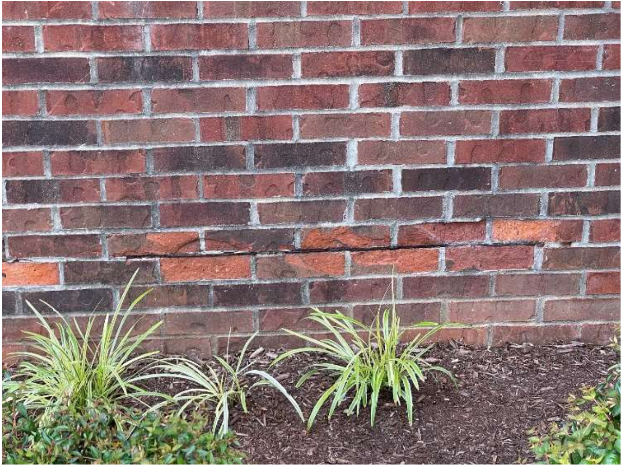
Figure 16 – Horizontal bed joint failure
