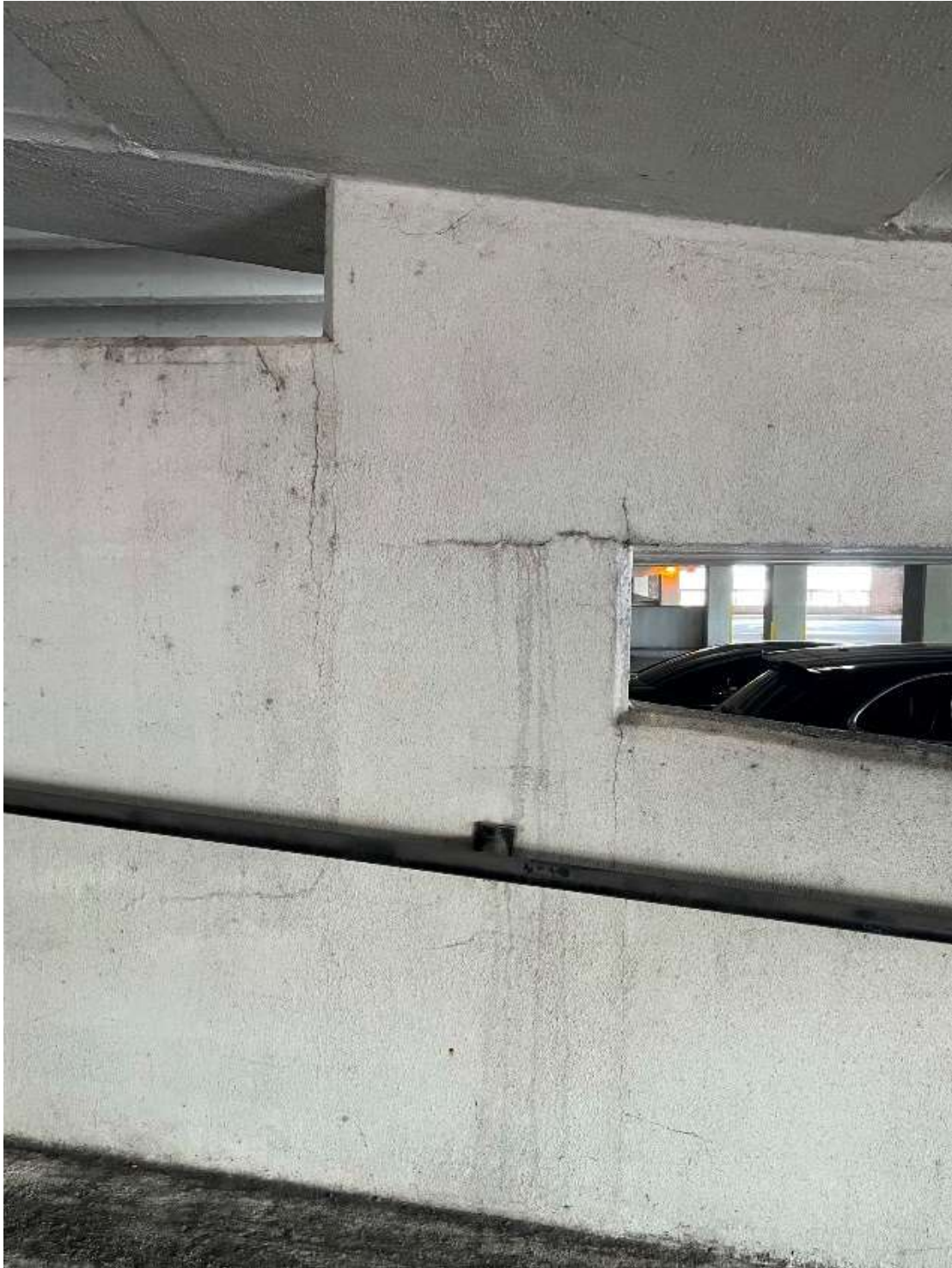
Figure 2 – Hairline crack at cold joint
