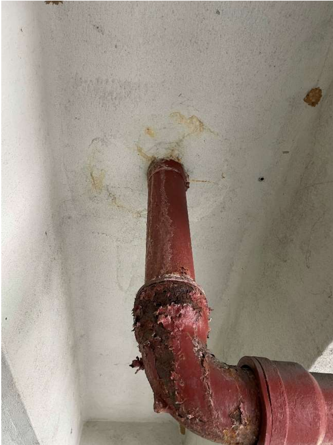
Figure 3 – Rust coming from drain penetration and corroded elbow
