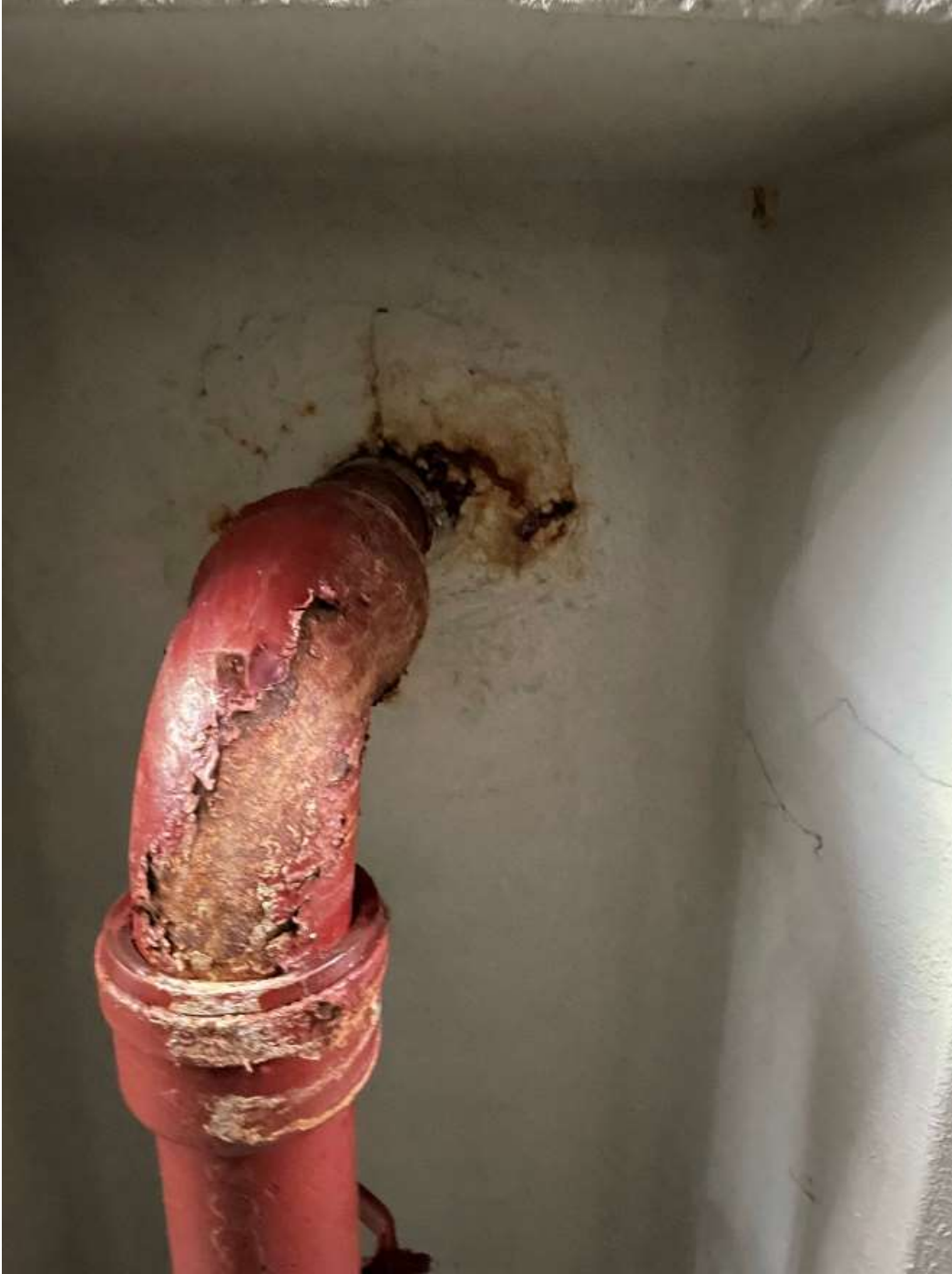
Figure 4 – Rust coming from drain penetration and corroded elbow
