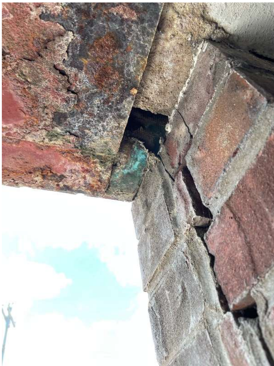
Figure 12 – Corroded lintel and brick veneer crack
