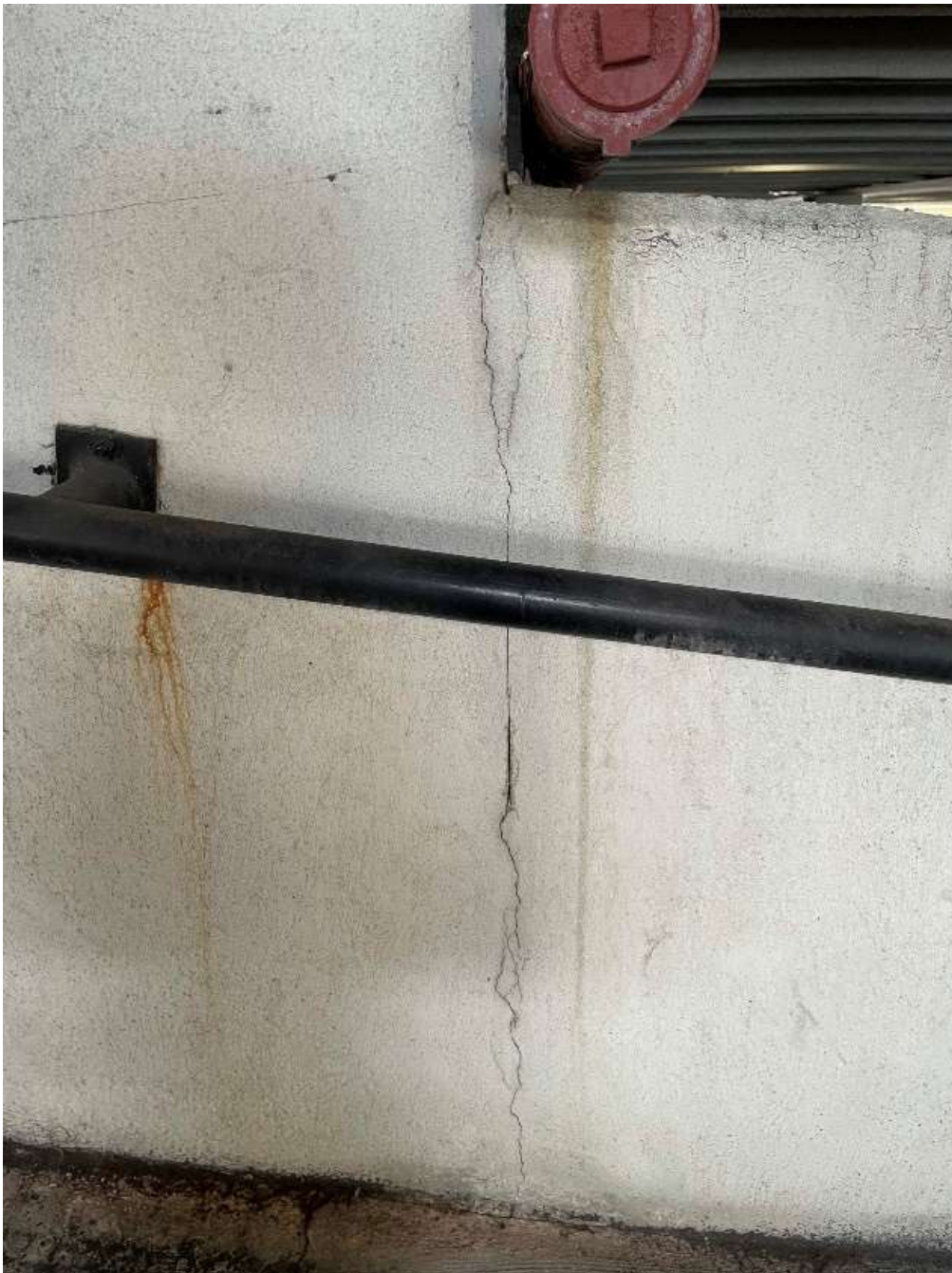
Figure 1 – Hairline crack at cold joint
