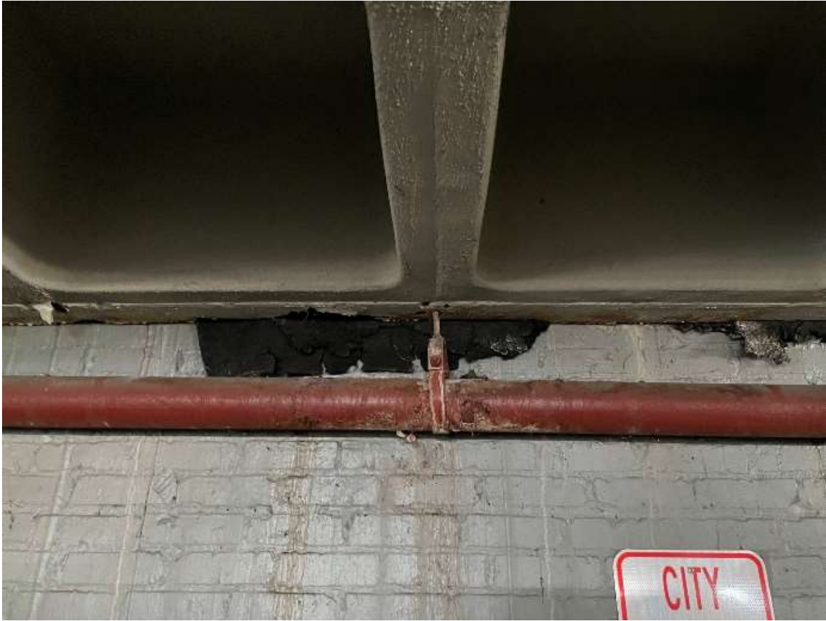
Figure 6 – Expansion joint filler material hanging from joint
