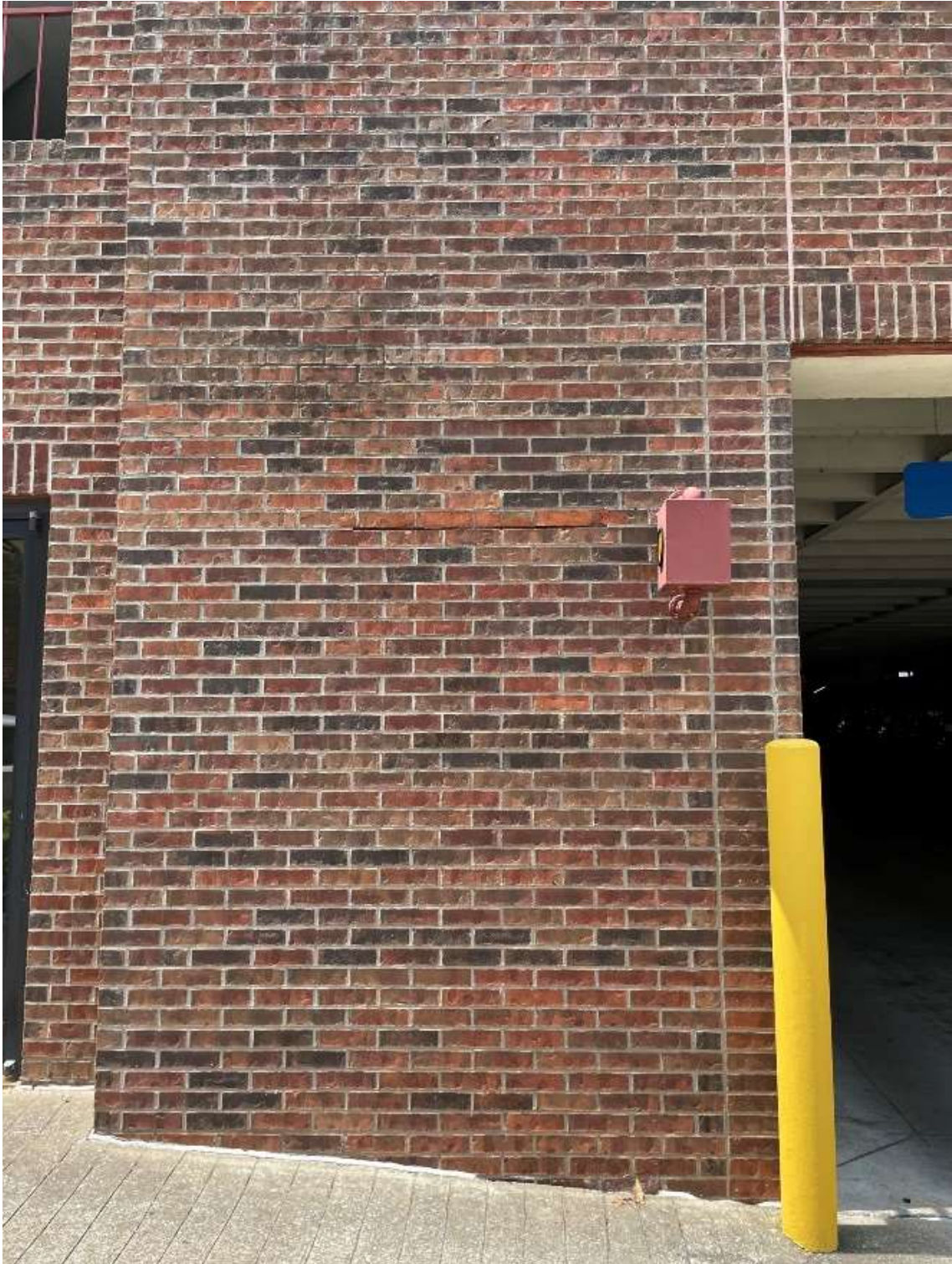
Figure 14 – Horizontal bed joint failure
