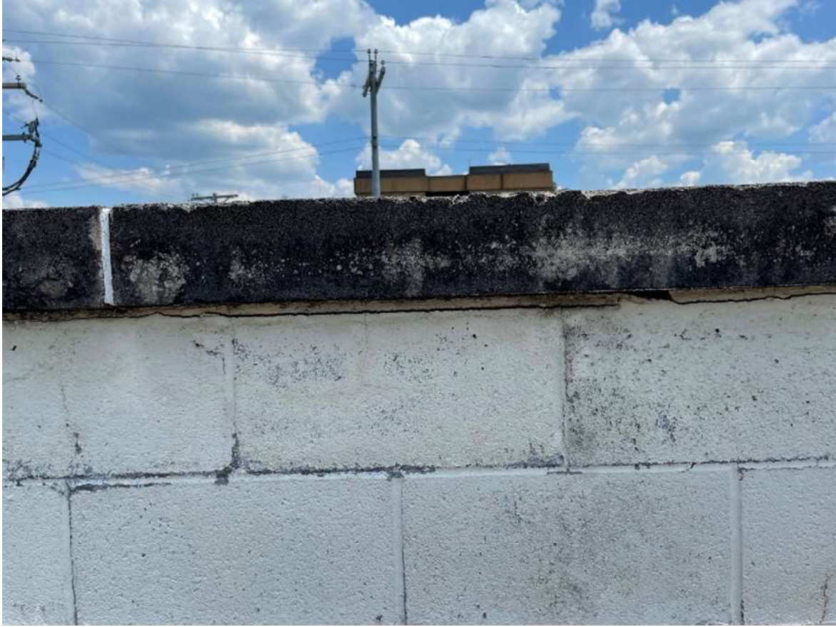
Figure 9 – Capstone bed joint crack
