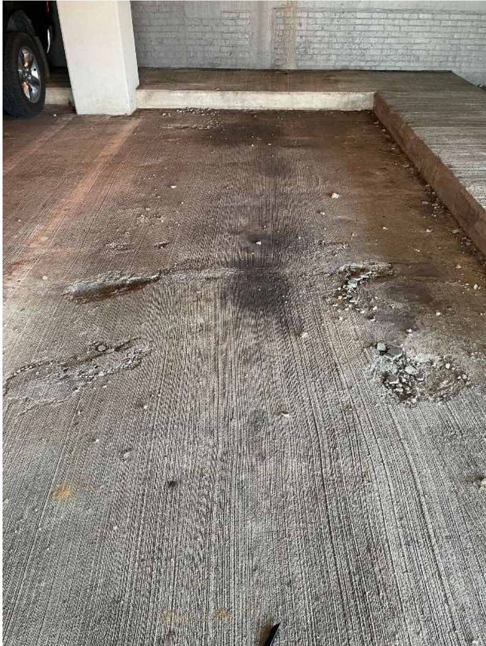
Figure 5 – Parking Space concrete spalling
